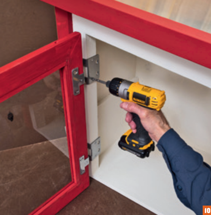
10. Add the door glazing and reinstall the door after finishing the structure.
